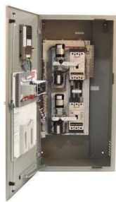
MC Auto Transfer Switch
