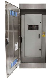
Medium Voltage Metal Enclosed Switch
